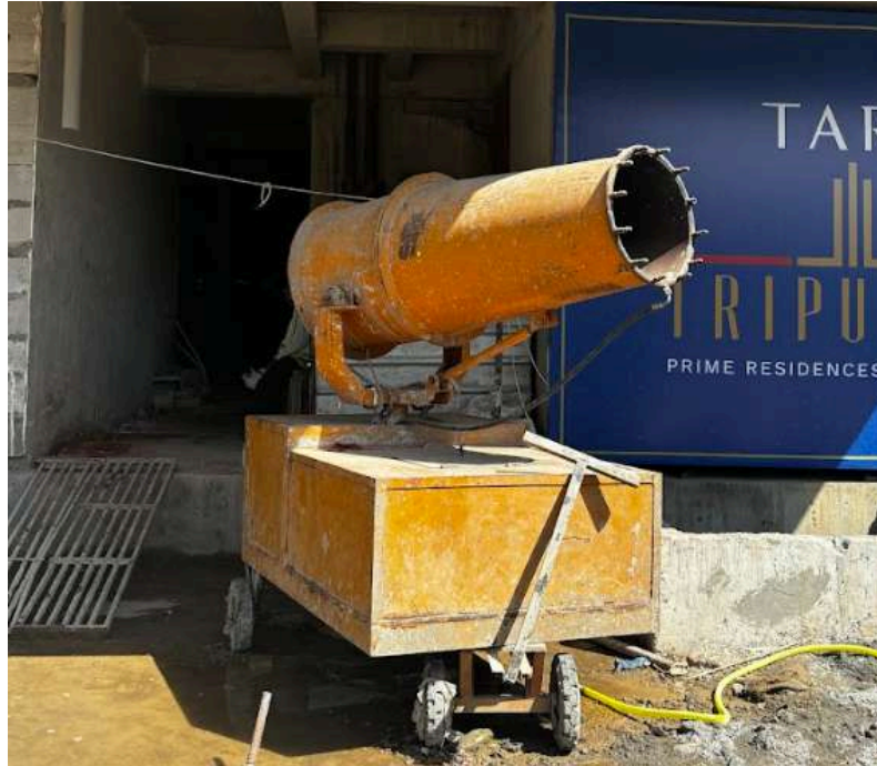
Figure 2. Anti Smog Installed at the Site
